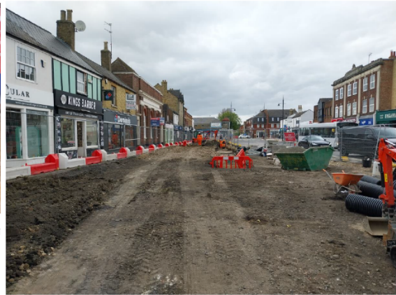
Asphaltic road surface removed and excavation initiated for Broad Street West Side Footway
